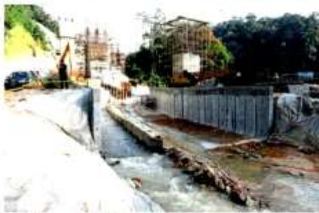
Geotextile is used at the EKVE project site to protect the soil.
